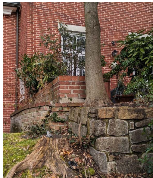
IMG. 14-720 Biological Growth and Vines Unit 14
