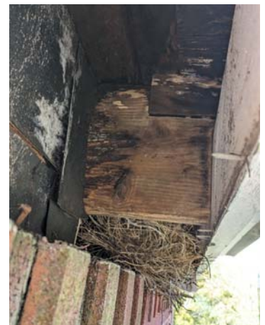
IMG. 7-650 Deteriorated Cornice
