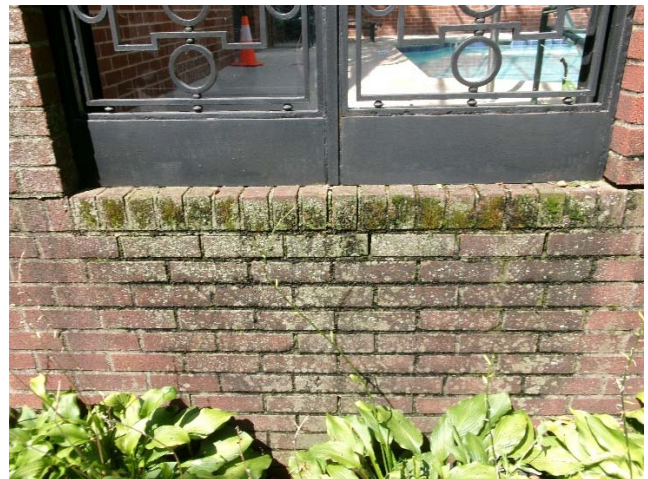
IMG. P-730 Biological Growth & Wash-Out Mortar NW Corner
